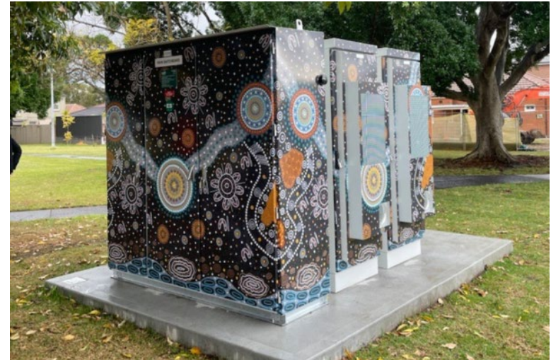
Source: Ausgrid (2023), Community Battery Pilot
