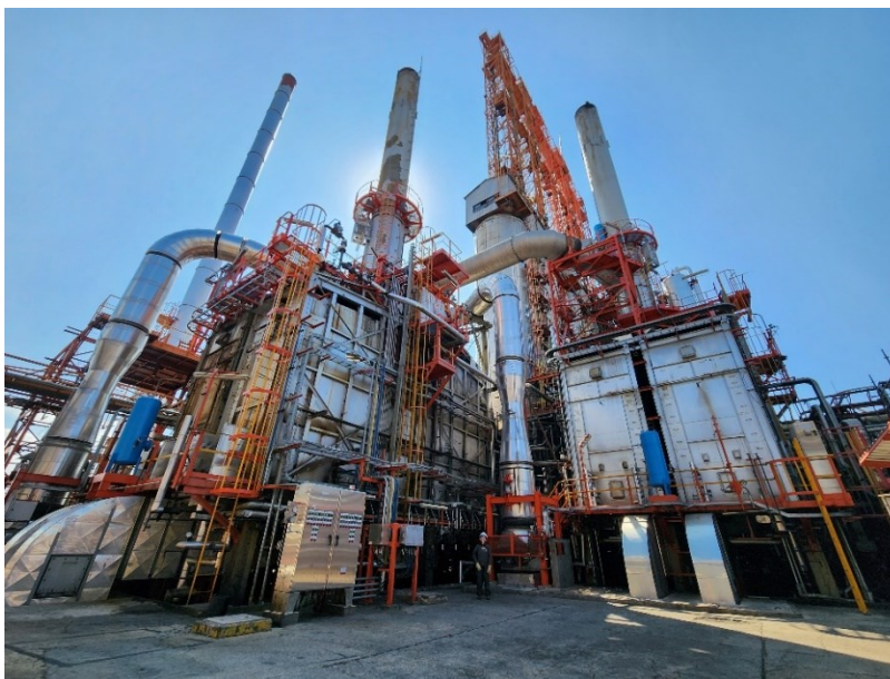
Figure 9 – Coker I Furnaces
