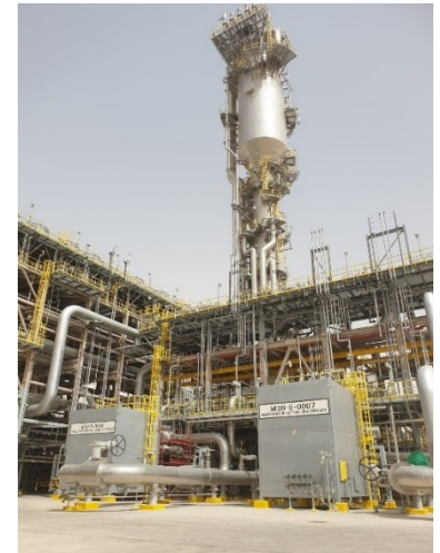
Figure 2: Ethane Recovery Unit
