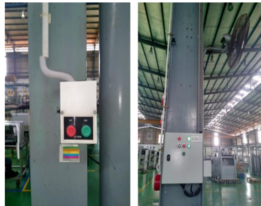
Installed fan controlling system in the production sector.
