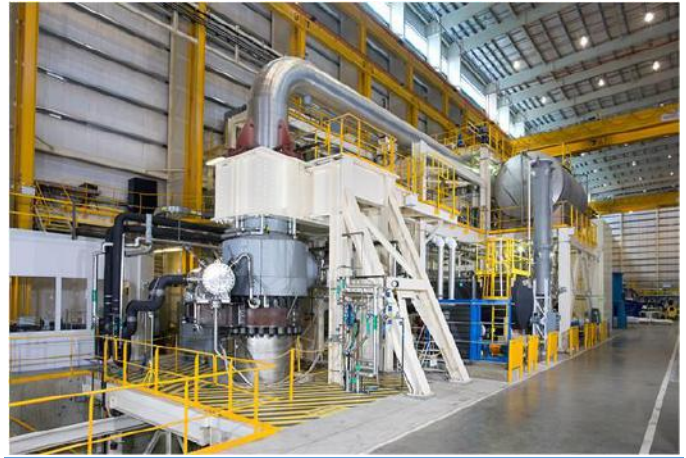
AP1000 RCP in Test Loop
