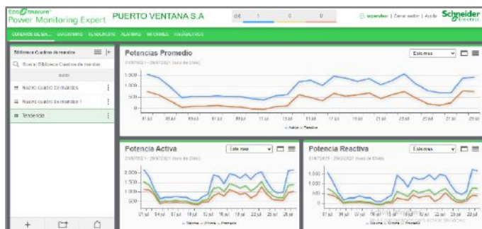
Figure 5: Screen of Power Monitoring Expert for energy data analysis
