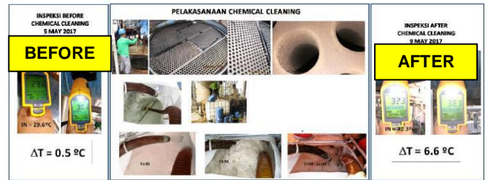
Figure 6. Monitoring energy efficiency on evaporator
