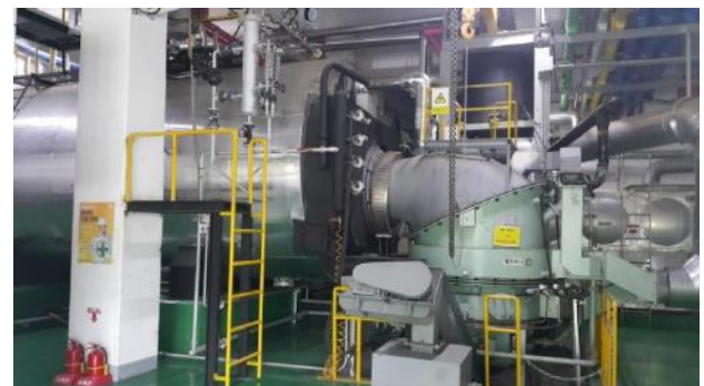
Fig. Wood pellet boiler of Laundry Factory
