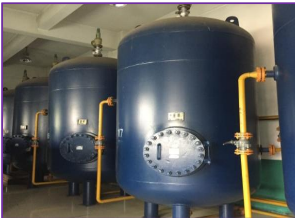
Centralized control transformation of air compressor station
