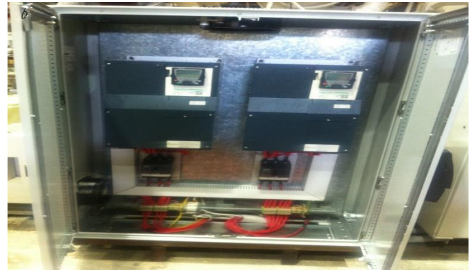
Figure 4: Installed VSD panel
