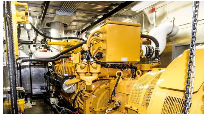
Photo 2: Inside the CHP engine room
